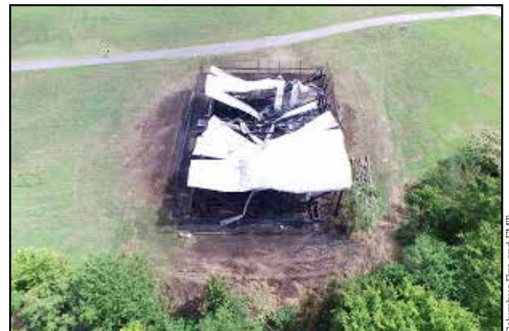
Burned out CWNM shed from the air.
