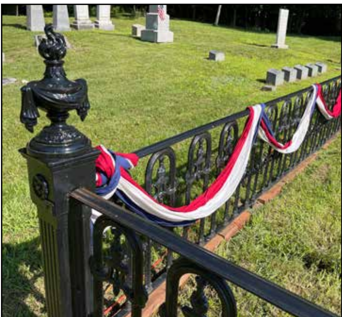
A new finial urn and a view of some new fencing that was re-created to replace lost and damaged parts.
